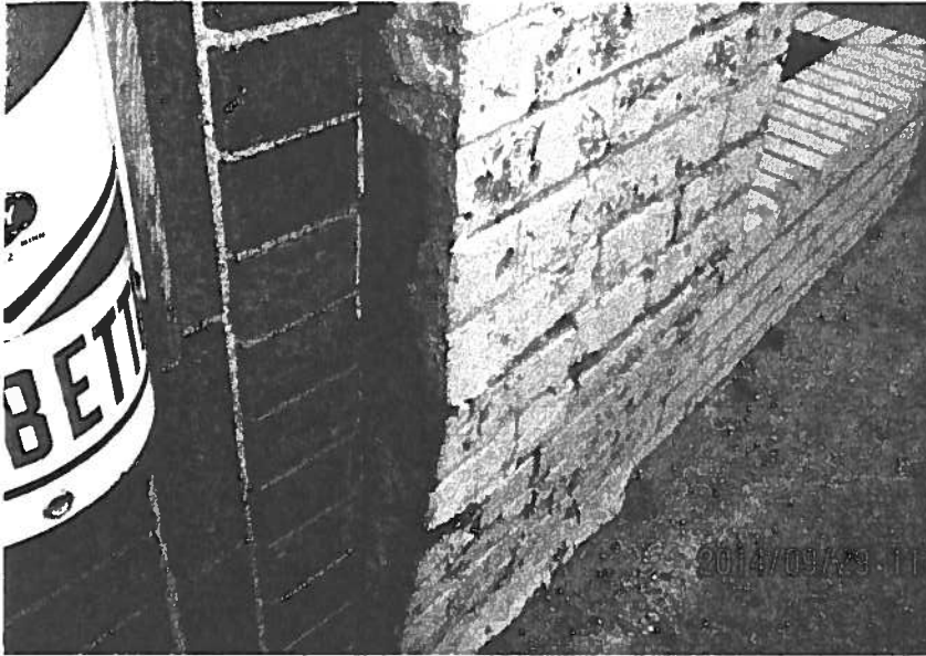
Other side of column shows like displacement. This area is open to water infiltration and further damage by freeze/thaw cycles.
