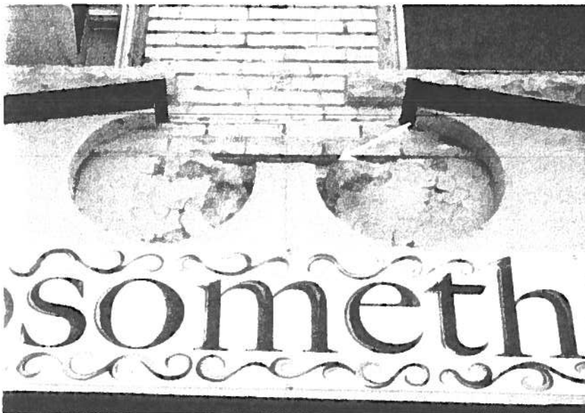
Some additional damage can be seen in the center of the pediment detail. This repair is not within scope of the emergency repair.
