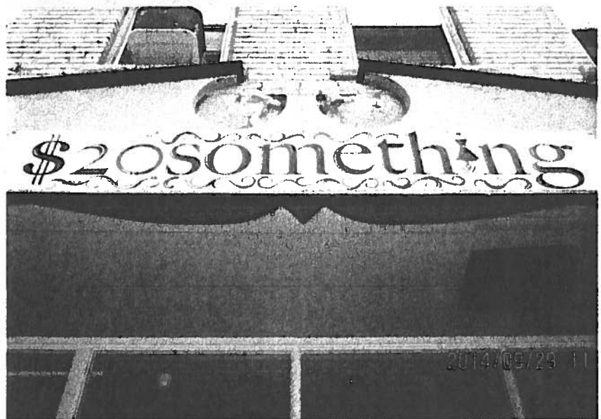
Pediment and some of the overhang will be removed to access the underlying framing to get positive placement of the shoring.
