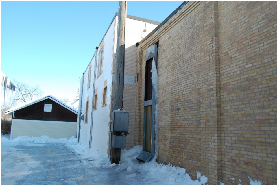
Facing SE: evidence of water damage
